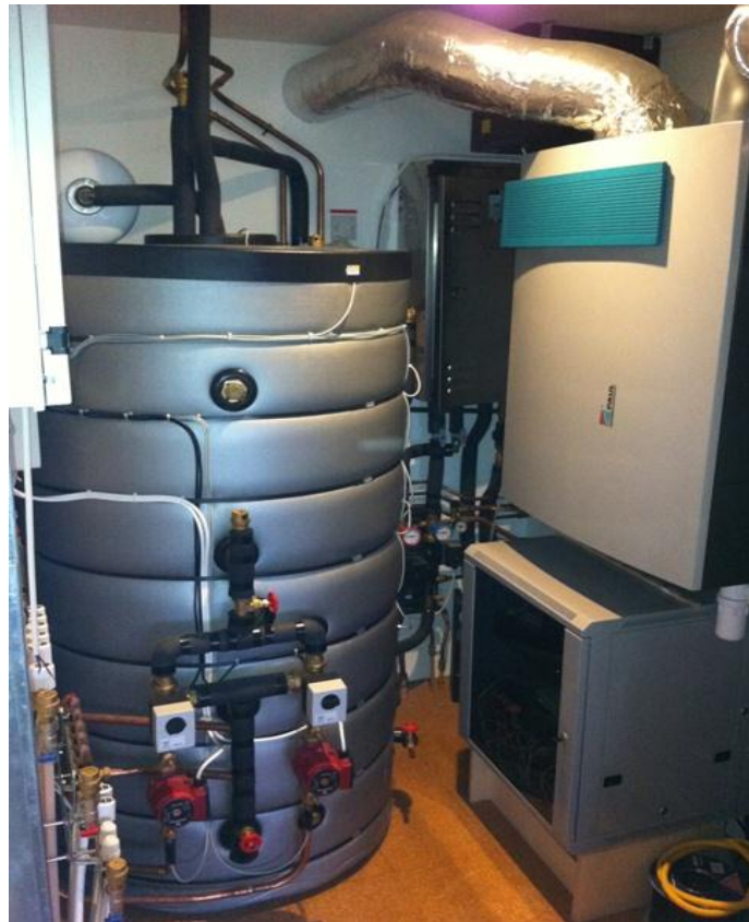
Figure 3-7: Heat Exchange Unit in Dwelling
