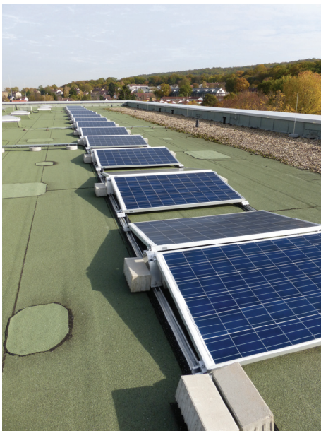
Figure 11: PV panels on the roof of the Solitude Gymnasium in east-west orientation and with low inclination.
