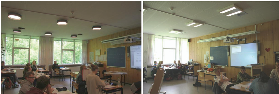
Figure 10: Two types of LED light fixtures in the renovated Hedegårds School in Ballerup.
