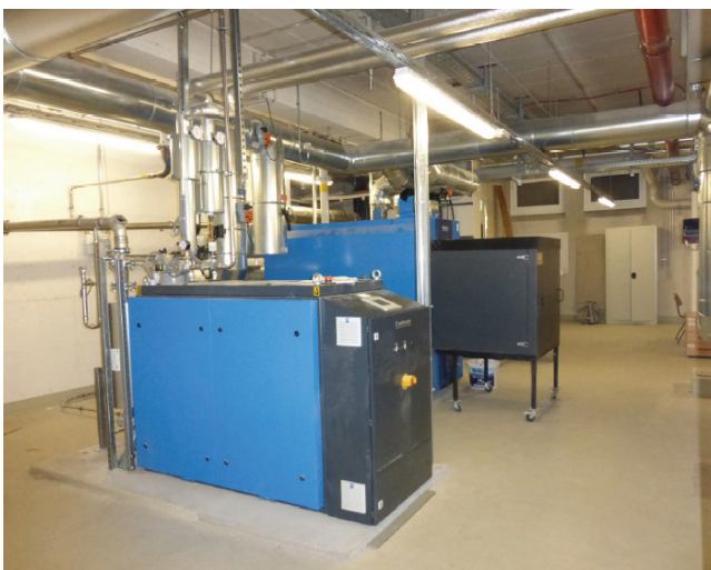
Figure 7: The combined heat and power unit and one of the gas boilers kept as back-up in the Solitude-Gymnasium Stuttgart.
