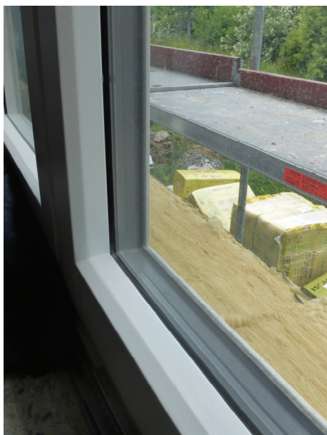
Figure 4: Triple-glazed window in the School of the Future demonstration building Solitude-Gymnasium, Stuttgart.
