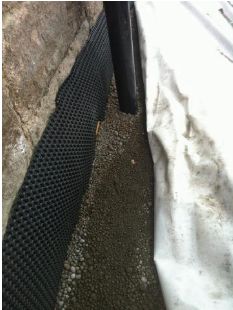
Figure 6: Combined digging for drainage, exterior insulation of walls to the ground and collector pipes at the School of the Future school in Drammen.
