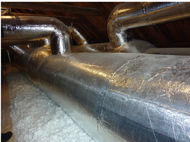
Figure 3: 30 cm mineral wool (flock) insulation on the ceiling to the attic at the Brandengen School in Drammen, a School of the Future demonstration renovation. The ventilation pipes received a thick insulation as well.
