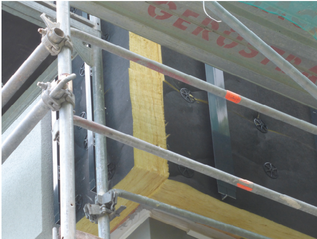
Figure 2: 18 cm mineral wool insulation on the external wall of the Solitude Gymnasium Stuttgart.
