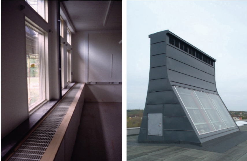
Figure 12: In the Tanga School, Sweden, outside air is supplied through air intakes in the exterior walls into a stub-duct hidden behind a bench (left). The fresh air is preheated using convectors under the stub duct. The exhaust air is extracted on the opposite side of the room into vertical ventilation ducts leading to solar chimneys (right) installed on the roof with leeward outlets and assisting exhaust fans (Source: [5]).
