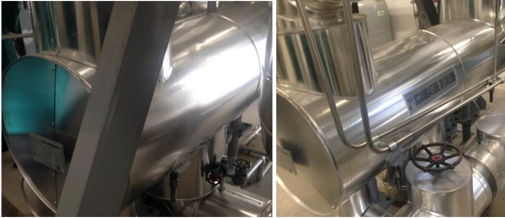
Figure 15. Steam-water heat exchangers (HX n° 1, left and HX n° 2, right). Source: Tecnia
