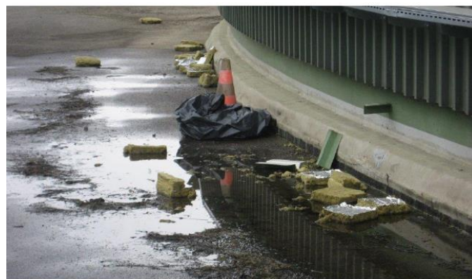
Figure 39. Envelope of the existing oil tank at RAG and its heat insulation. Source: RAG.
