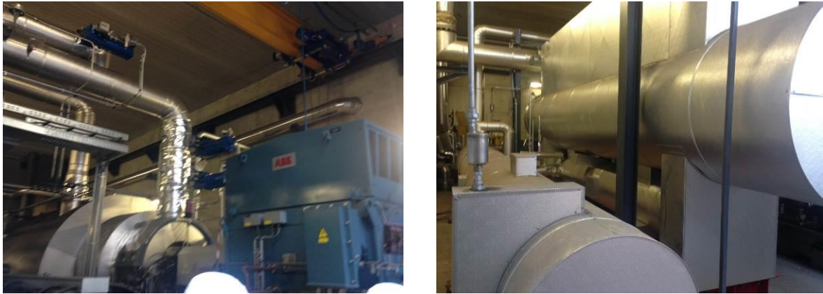
Figure 11. ORC Turbine and Generator (left) and ORC Evaporator shell and Condenser. Source: Tecnalia
