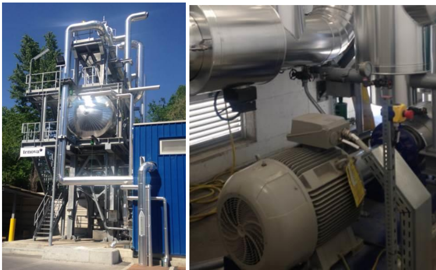
Figure 16. Flash Tank and Condenser in the upper side (left); water circulating pumps to Condenser (right). Source: Tecnia
