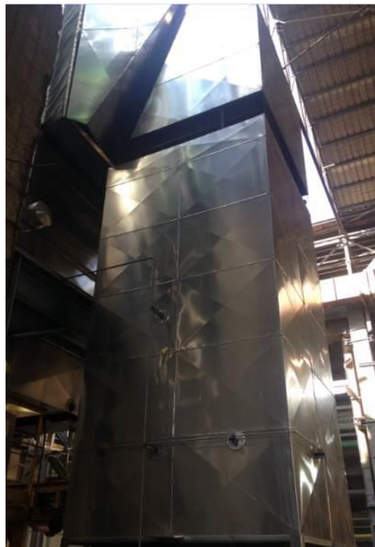
Figure 3. Flue gas duct inlet to WHRU from EAF. Source: Tecnalia
