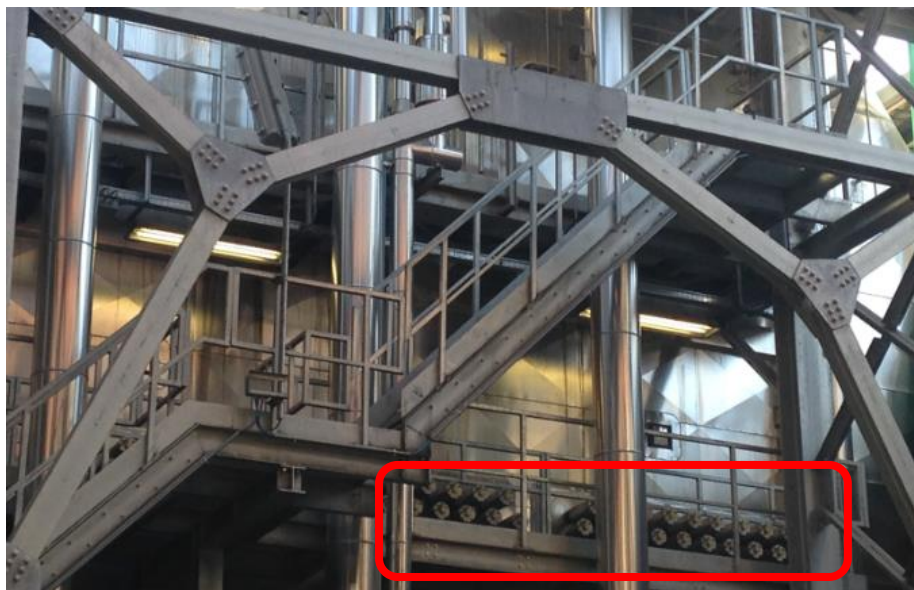
Figure 5. Pneumatical WHRU cleaning system. Source: Tecnia
