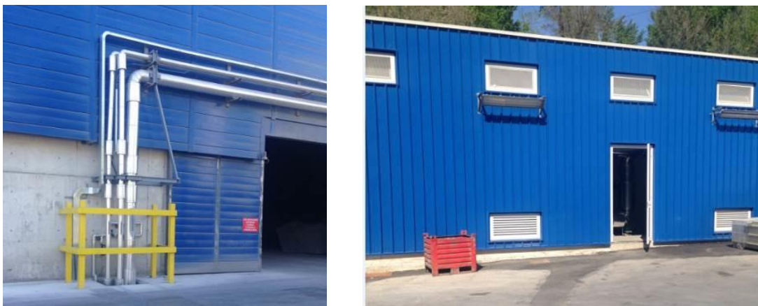
Figure 14. Steam pipes to DH system (left) and DH system equipment cabinet (right). Source: Tecnalia
