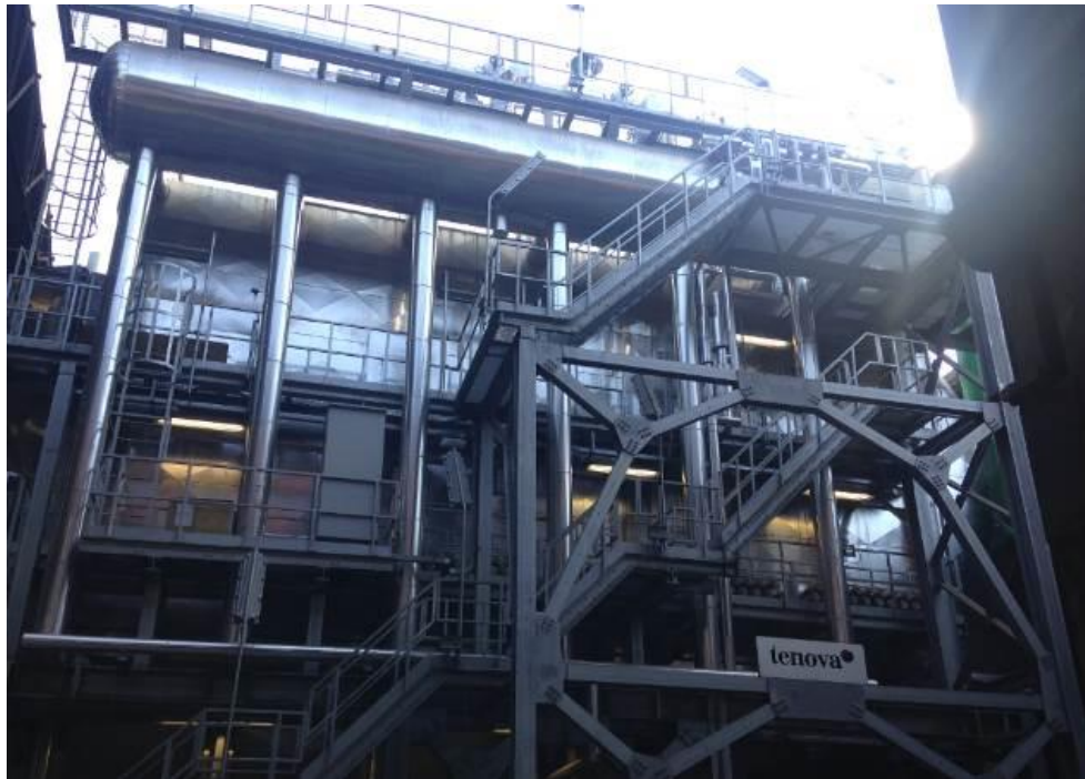
Figure 4. Waste Heat Recovery Unit, formed by one Economizer (right side), four Evaporators (left side) and one Steam Drum at the top. Source: Tecnia
