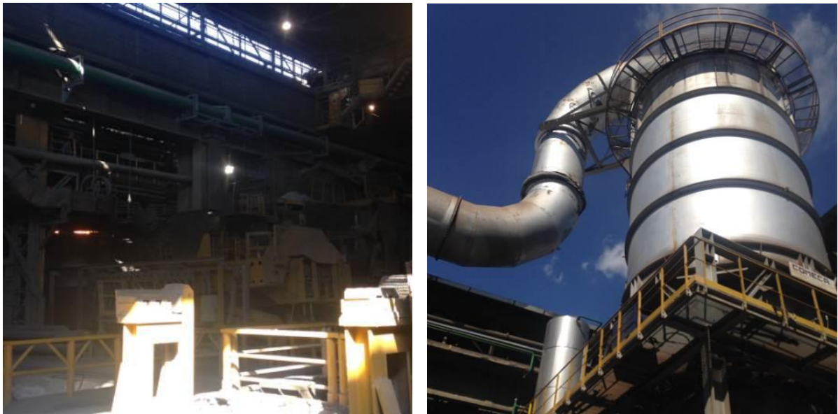
Figure 2. EAF (left) and outlet duct from WHRU to Quenching Tower (right). Source: Tecnalia.
