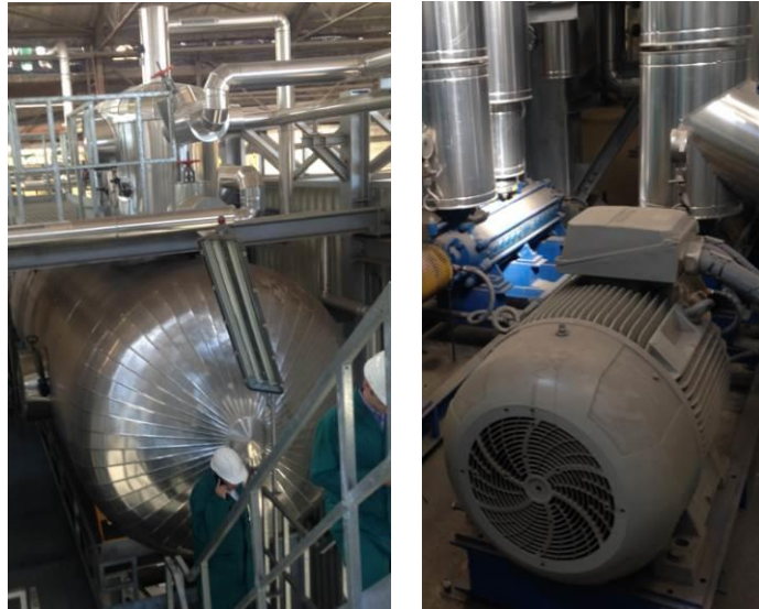
Figure 7. Feed water tank and demister in the top part (left) and one of the boiler feed water pumps (right). Source: Tecnalia
