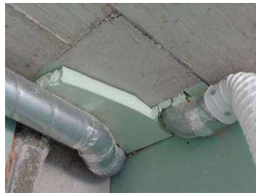
Extraction tubes in kitchens are insulated from the rest of the elements to avoid the transmission of noise and vibrations.
