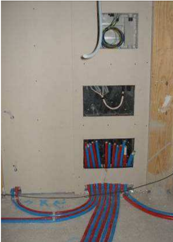
Pipes for heating (March 2013)
