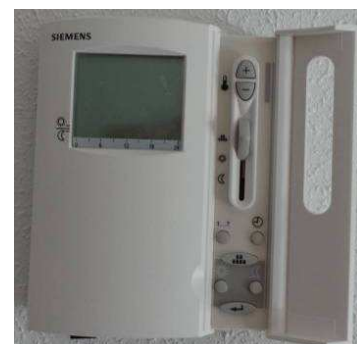
Heating thermostat in the living room
