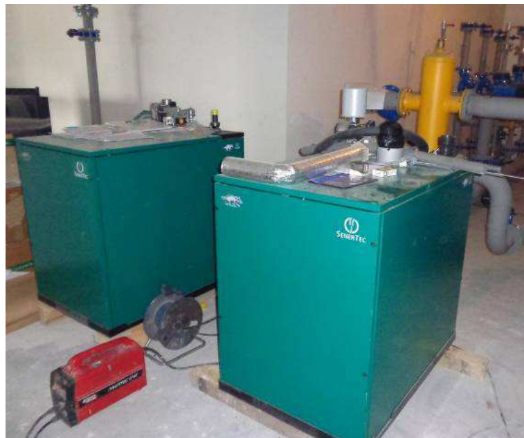
Cogeneration engines in the boiler room of A32 building
