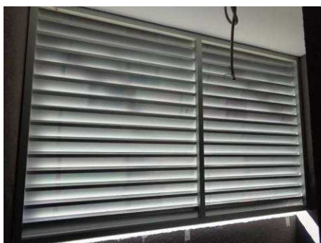
Ventilation grilles in the clothes drier area
