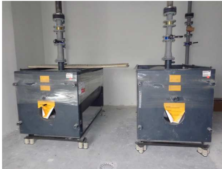
Condensation boilers in the boiler room
