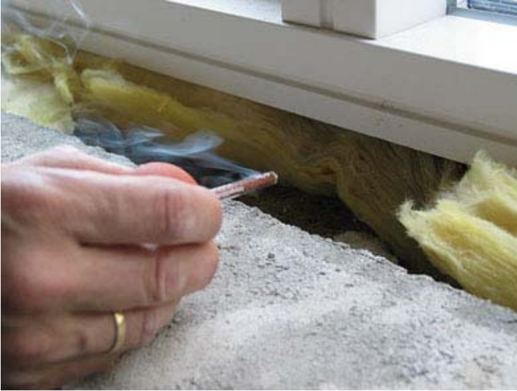
Fig. 2.6.1.2. The smoke test helps locate the place which is not complete by airtight.
