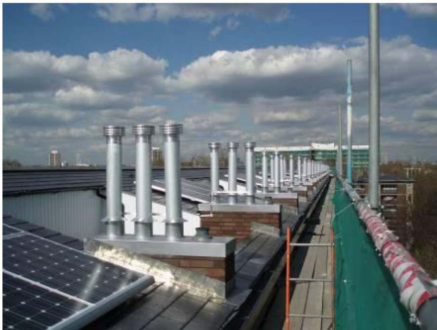
Figure 3: PV Panels at the Mursell Estate
