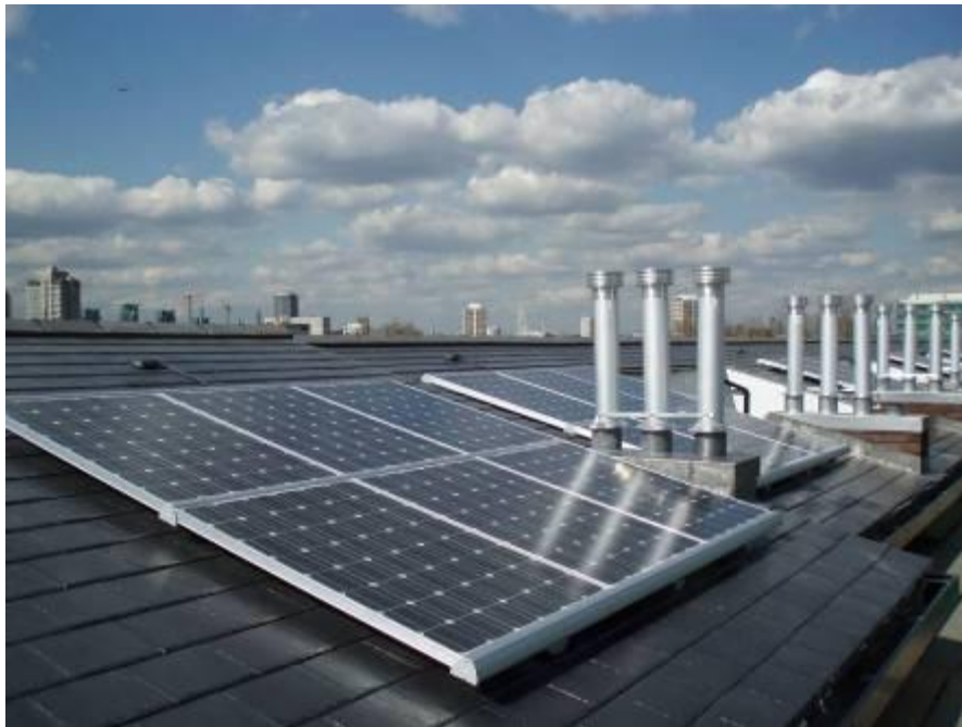
Figure 2: PV Panels at the Mursell Estate
