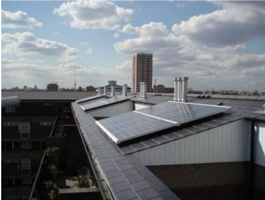
Figure 4: PV Panels at the Mursell Estate
