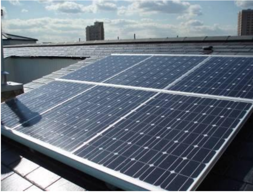
Figure 6: PV Panels at the Mursell Estate
