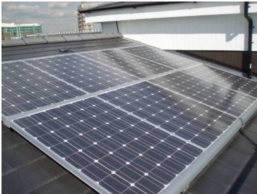
Figure 5: PV Panels at the Mursell Estate
