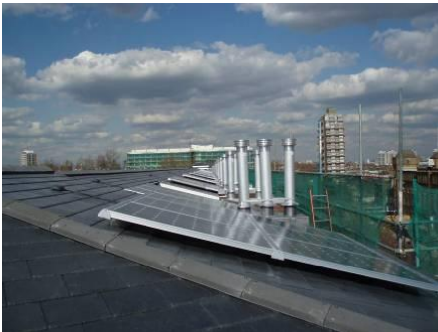
Figure 1: PV Panels at the Mursell Estate
