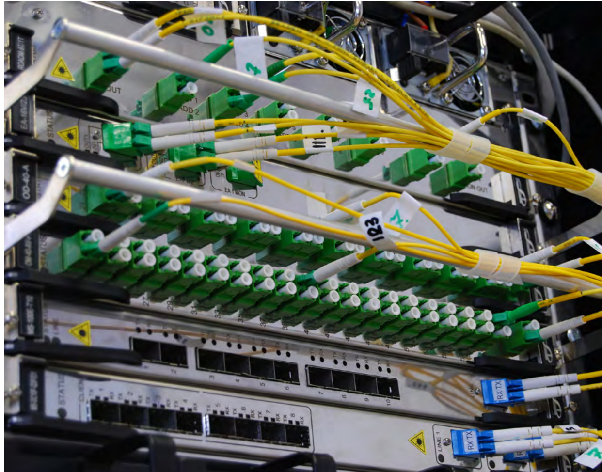
Optic-fiber telecommunication equipment in rack ©Kirill Sh, Unsplash
