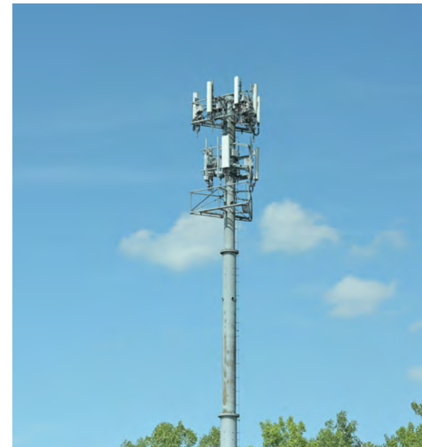
Telecommunication tower ©Nathan Anderson, Unsplash
