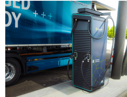
Electric truck charging ©Netze BW, Unsplash
