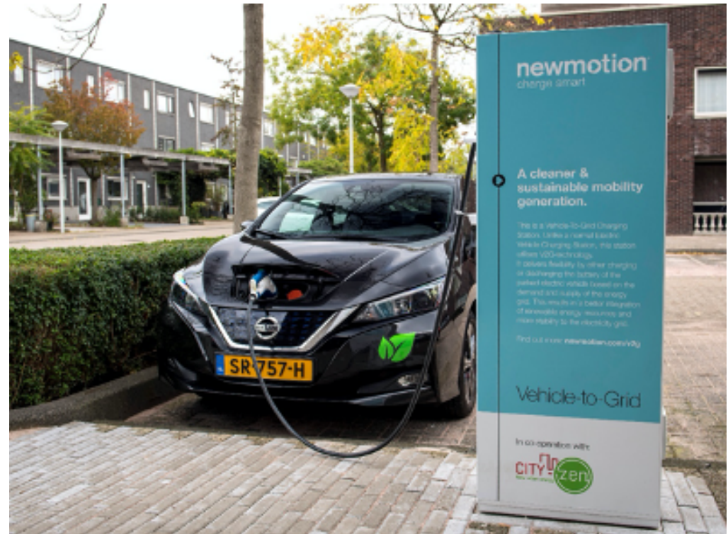
Bi-directional V2G charging station installed for the City-zen Project VPP pilot. ©Alliander
