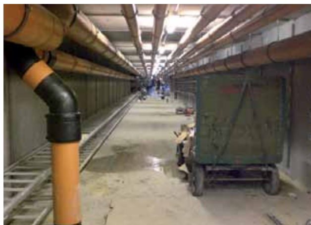
Image 5.3: Biogas Plant in Måbjerg (DK)
